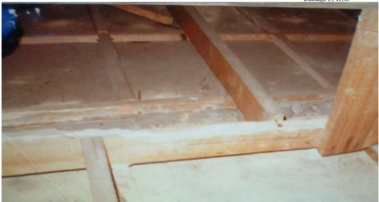
Damage by Hylotrupes
